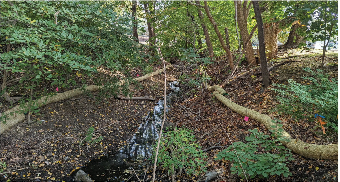
Erosion control waddle (12") installed just above the wetland line marks the limit of invasive species management and slows any erosion from entering the wetland
