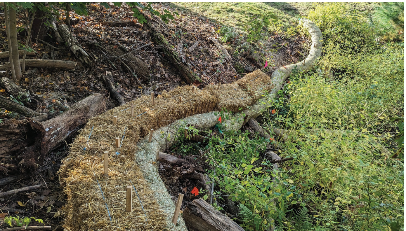
Straw bales placed along the top the straw waddle to further protect from sediment entering the wetland in certain areas
